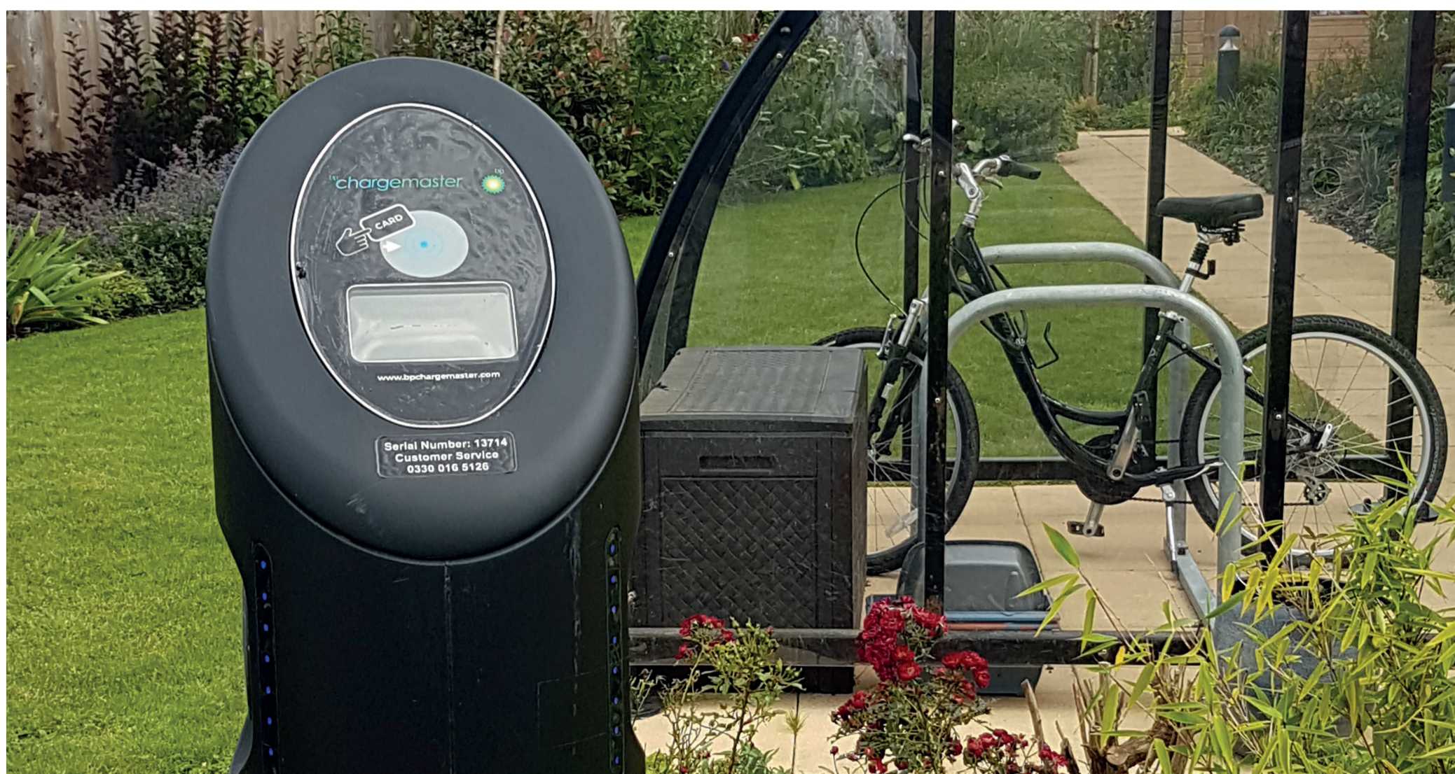
EV charging unit
